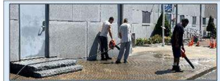
Under the supervision of Hardscape Instructor Dave Collins, participants replaced the large section of brick in front of our Middleton facility
